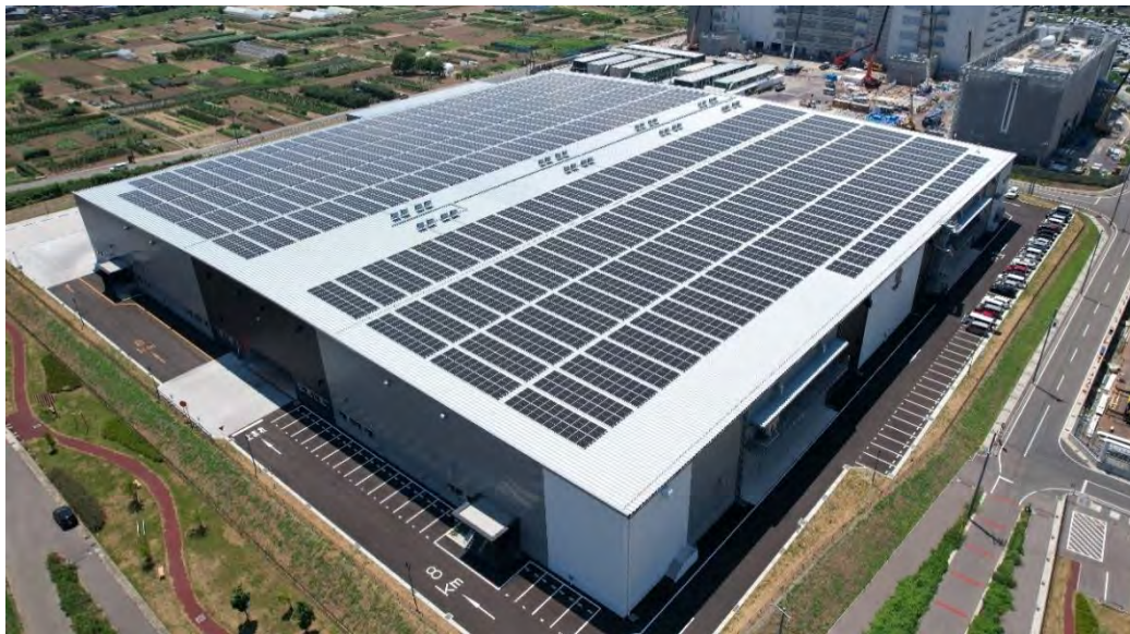
Solar power plant in Nagano
